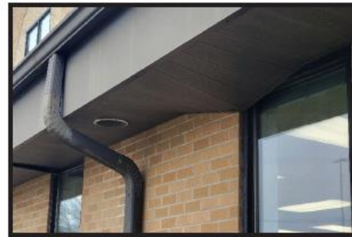
Damaged Exterior Increasing the Flow of Air Infiltration.
