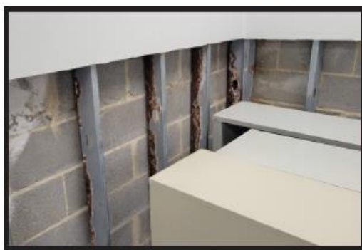
Interior Water Damage from Exterior at Below Grade Locations.
