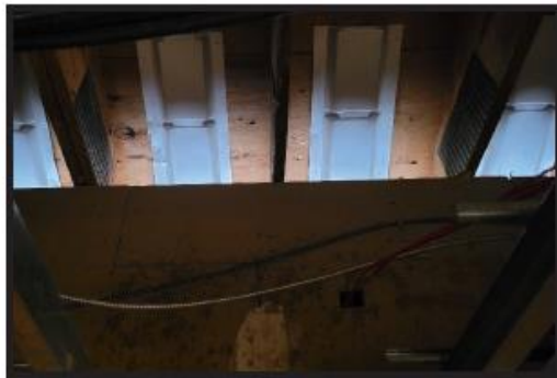
Photo Taken from the Interior Shows Eaves Wide Open to the Outside.
