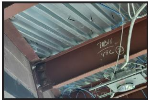
Poor Steel Connection (Knife Joint)
