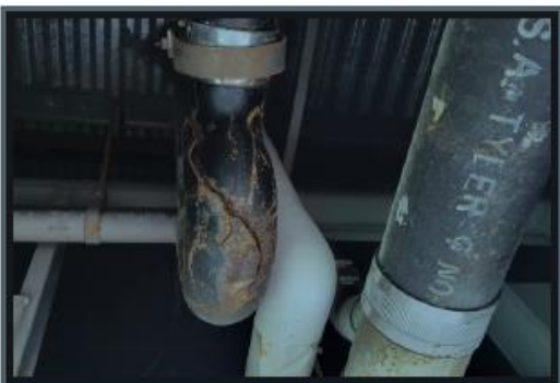
Broken Sanitary Drains in Need of Replacement.
