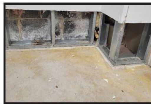
Exterior CMU Block in need of Damp Proofing at below grade locations.
