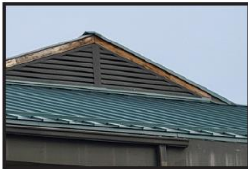
Louver and Fascia Trim in Need of Replacement.
