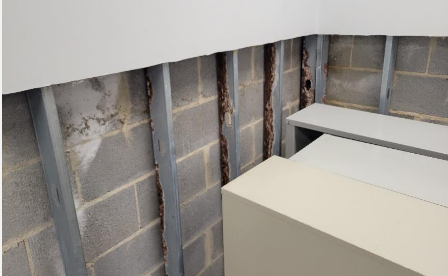
Interior Water Damage from Exterior at Below Grade Locations
