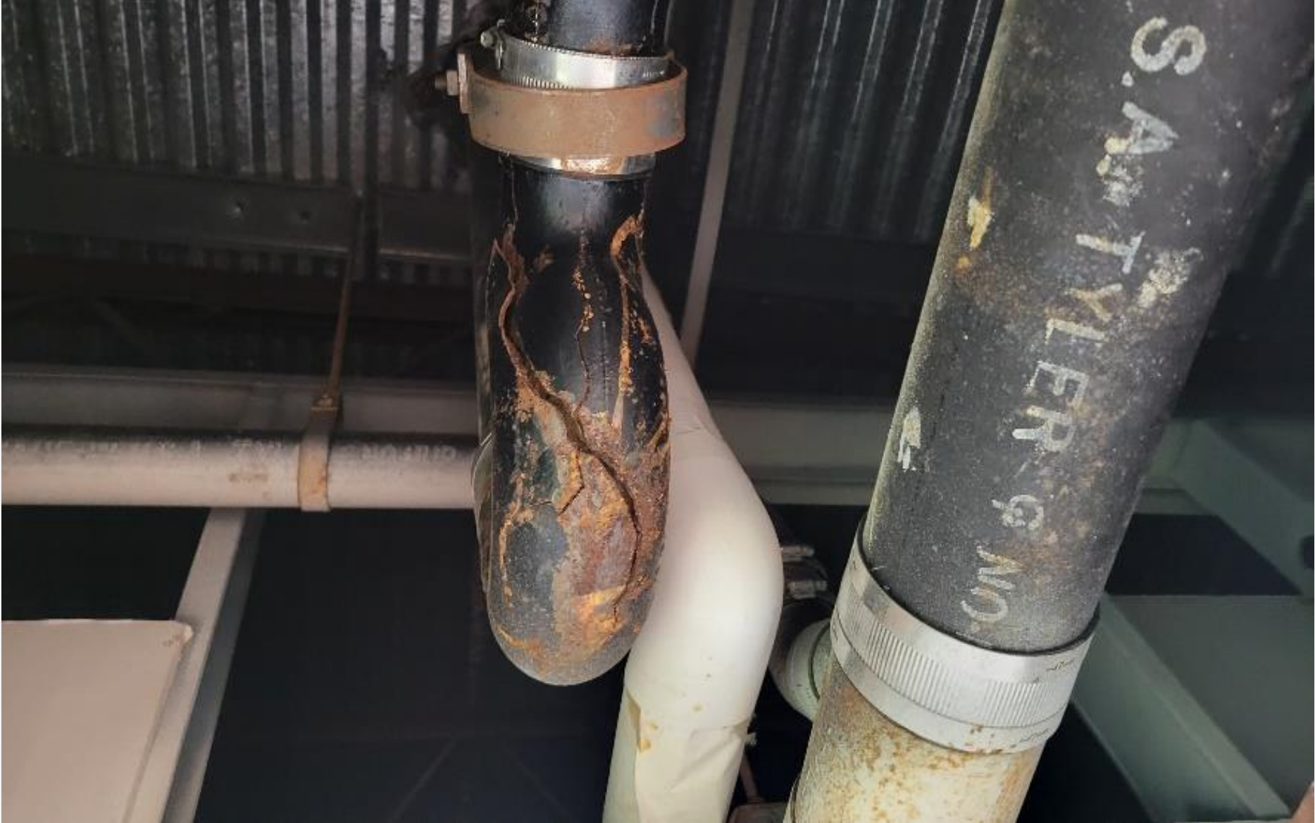
Broken Sanitary Drains in Need of Replacement
