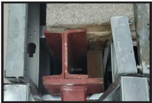
Structural Steel Concerns to be Addressed
