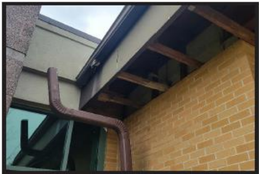
Exterior Soffits and Gutters in Need of Reconstruction / Replacement.
