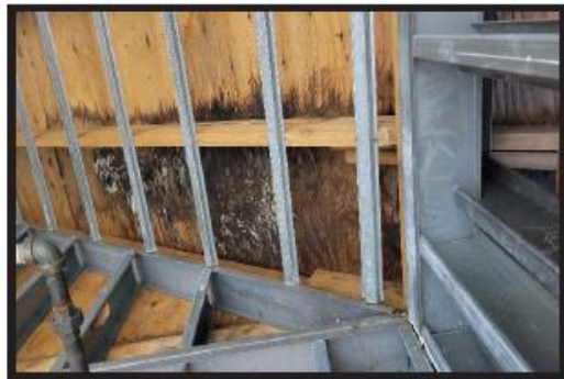
Wood Sheathing at Interior Roof Line in Need of Replacement. Water Infiltration Needs to be Addressed.
