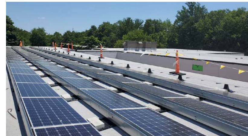
CRSD - Hillcrest Elementary School (Low Profile Solar Panels)
